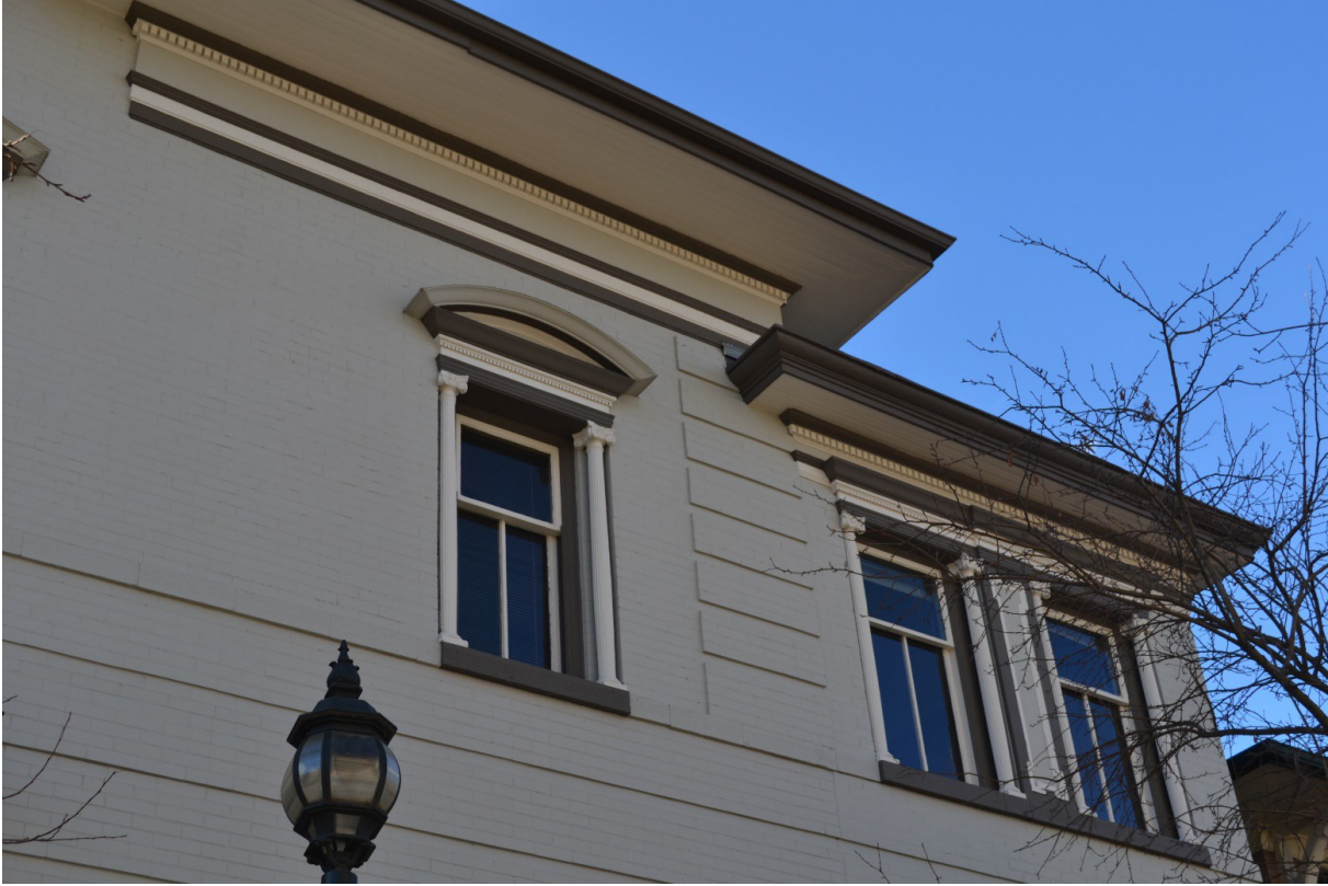
(Above) Rear Addition to the home, facing east. Quoins indicate where original corner was.
