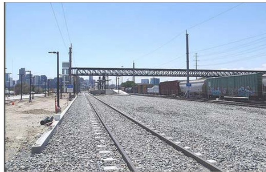
Bicycle/pedestrian bridge at the 41 st and Fox Station platform construction site (Source: RTD)
