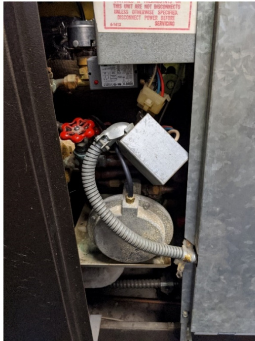
Figure 2: Typical CHW Valve
