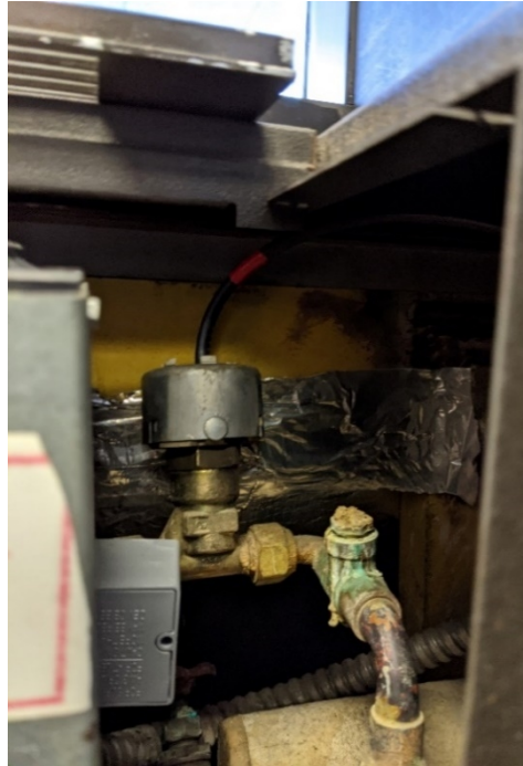
Figure 3: Typical HW Valve
