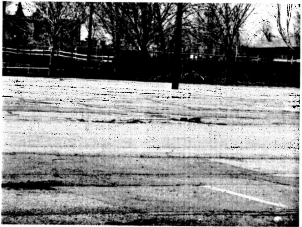
Patches of deteriorated pavement in interior parking lots
