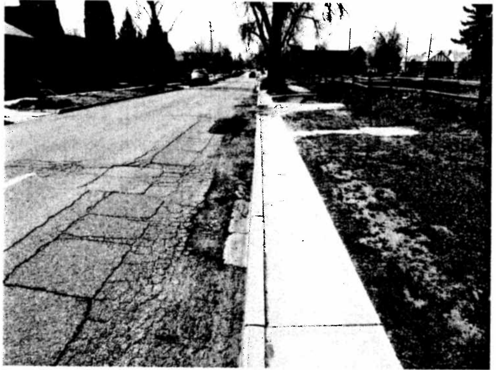
Deteriorated pavement in the public right-of-way
