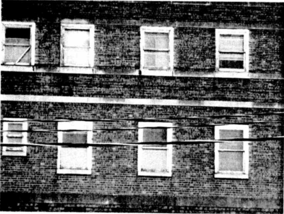
Windows on the Kuhlman Building were in disrepair
