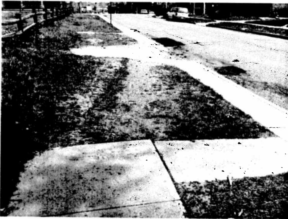
Sidewalk infrastructure will need to be rebuilt
