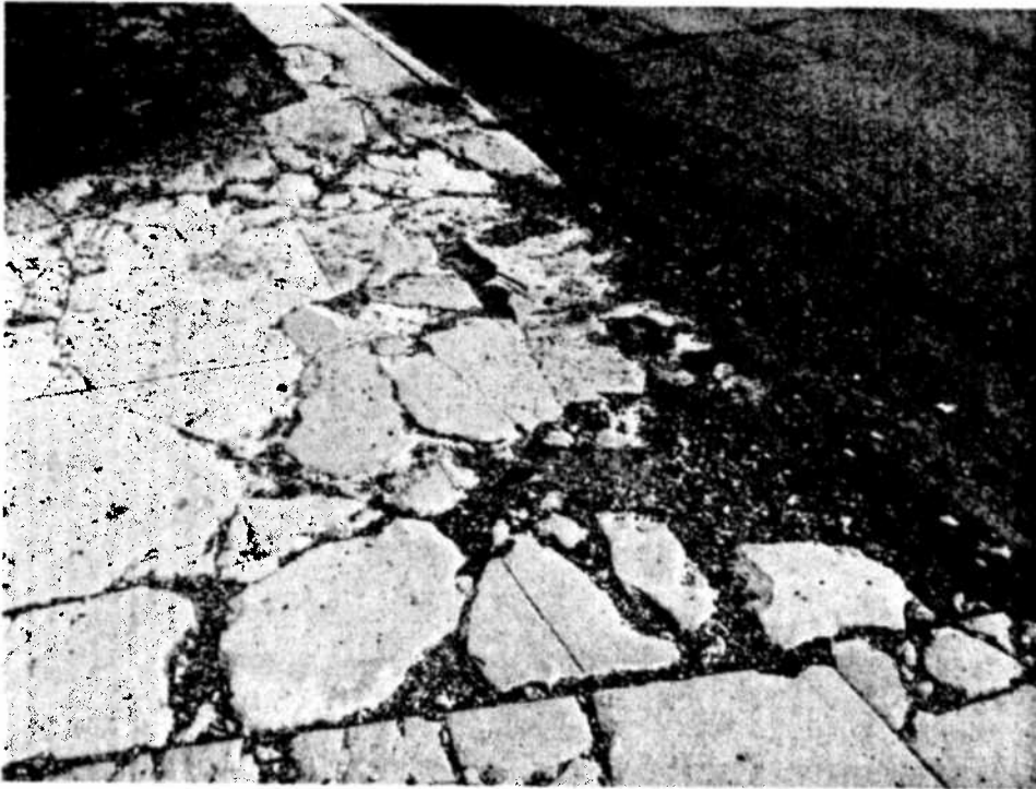
Deteriorated curb cut
