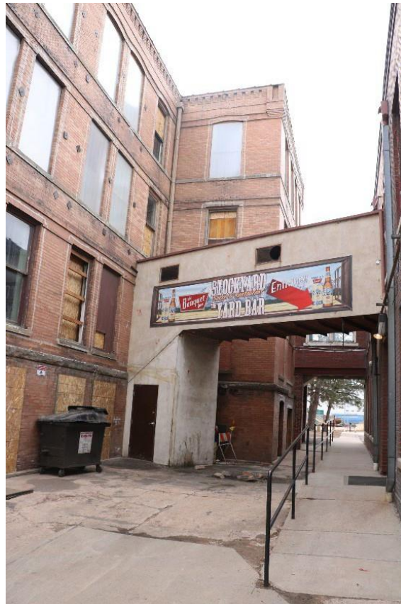
Walkway between 1898 and 1919 buildings, some boarded windows, and brick detailing Mead & Hunt photograph, November 2018
