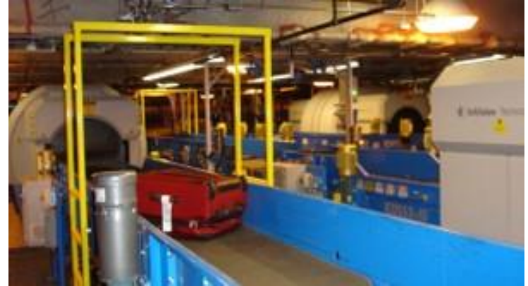
DEN's Existing EDS Equipment
