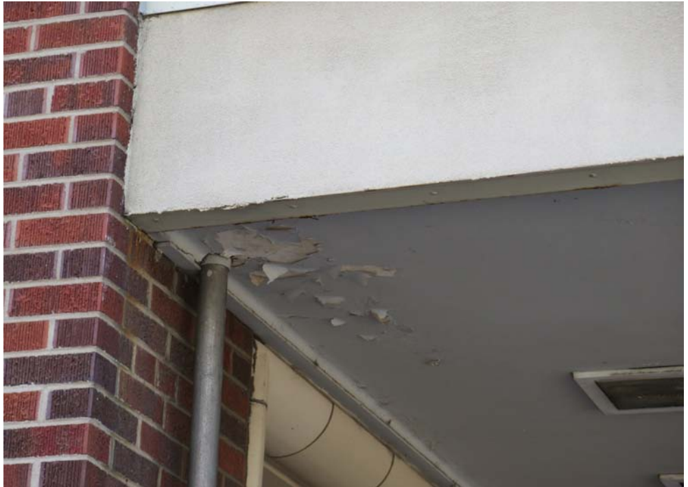
Peeling paint at Emily Griffith property
