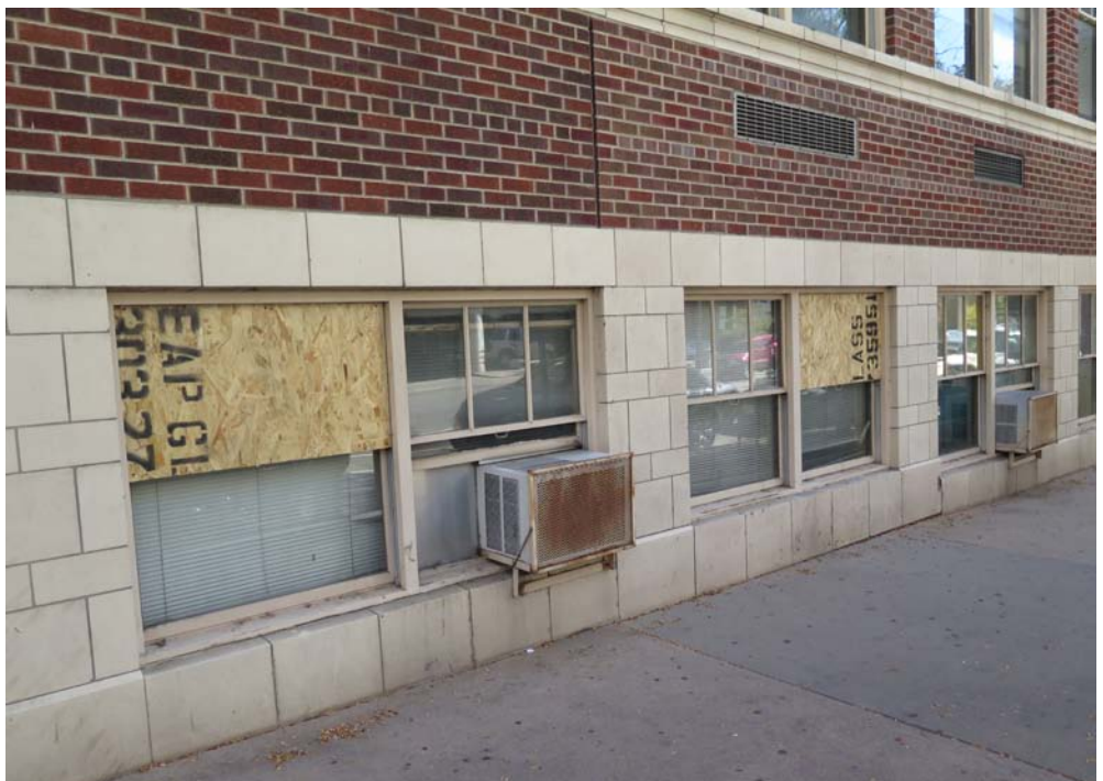
Broken windows at Emily Griffith property
