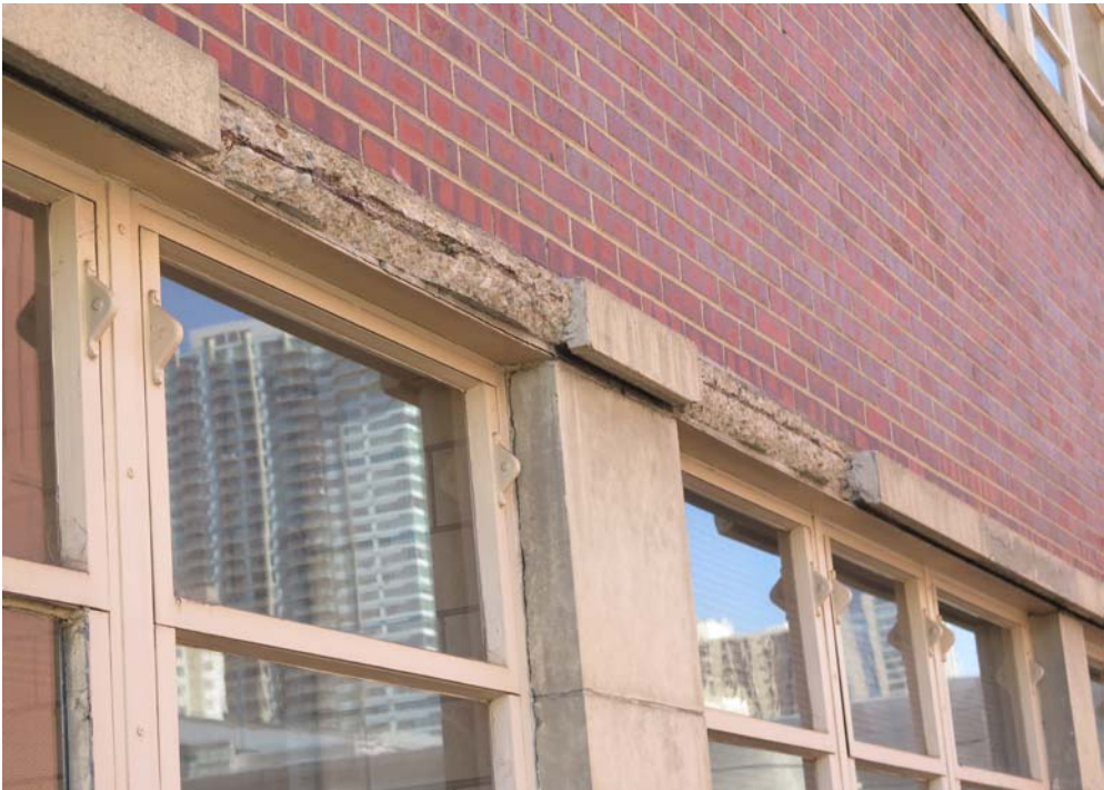
Deteriorated exterior elements above windows at Emily Griffith property
