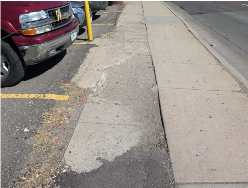
A sidewalk in degraded condition along Colfax
